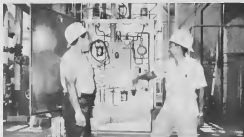
Pedro Tromp (at left) and Ramon Hodge adjusting the oil mist generator distribution pressure.
